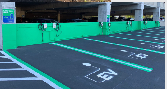
EV charging, Madisonville Operations Center, Cincinnati, OH
